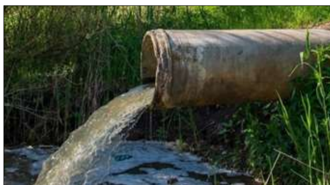
Waste water collection
