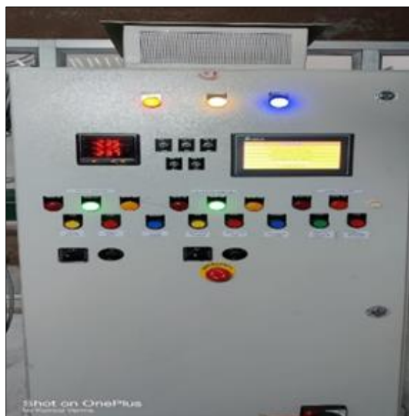
(c) Control panel
