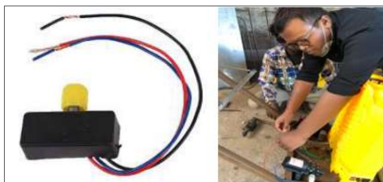
Fig 10: wiring connections of the battery and the pump and the solar panel.
