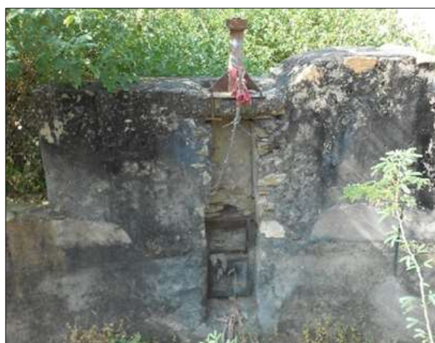
Fig 6: Damaged gate of RMC
