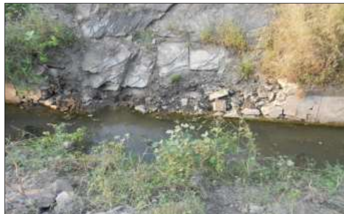
Fig 4: Damaged lining of RMC
