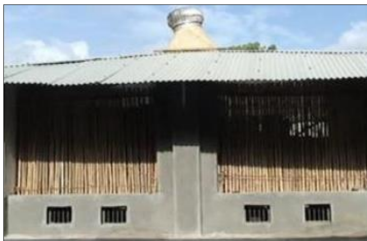
Plate 8: Turbine air ventilated storage structure
